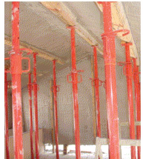
Photo 11: Place shoring on the underside of the floor and roof panels at intervals of 4-6'.
